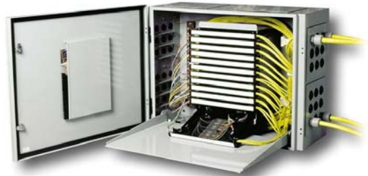
Front view of a loaded Telect 288-fiber splice vault.
