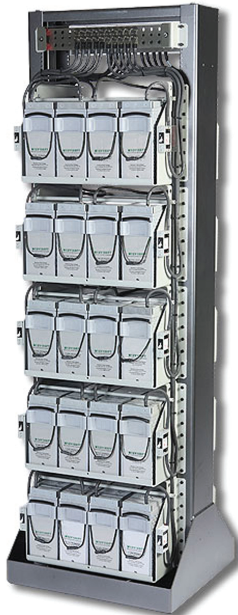
Figure 1: Example of a fully loaded five-shelf battery rack. This configuration holds a total of 20 batteries, providing a high-density, high-capacity solution for large-scale applications.
