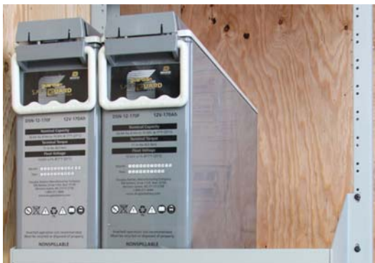
Equipment such as power distribution, connectivity (top photo) and batteries (bottom photo) can be part of a rack-mount application in a telco closet.
